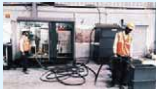
Photo shows filling of transformer oil at a manufacturing facility of Rajasthan Powergen Transformer Pvt Ltd
